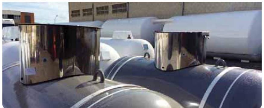
INSPECTION CHAMBERS ON UNDERGROUND TANKS
